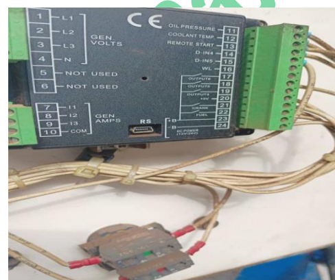
Existing 200kva Electronic
