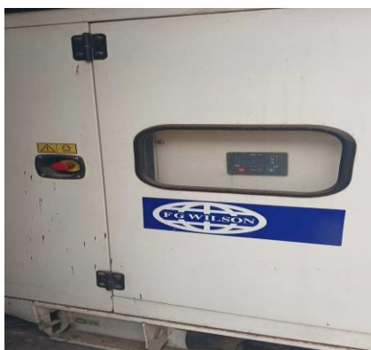
Existing 200kva Generator Board
